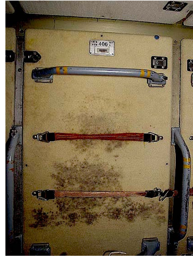
Mold growth on fabric panels on ISS from wet hanging towels
